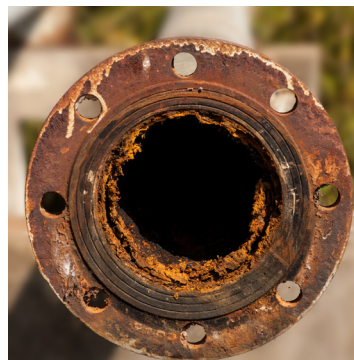
ID of corroded pipe sample
